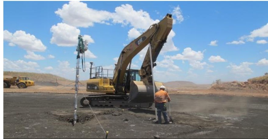
Instrument Tree Secured with Wire Stays
