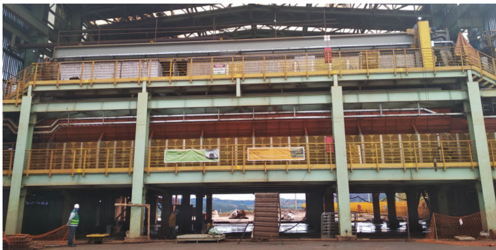
FIG 3 – Filter press installation for iron ore tailings treatment.
