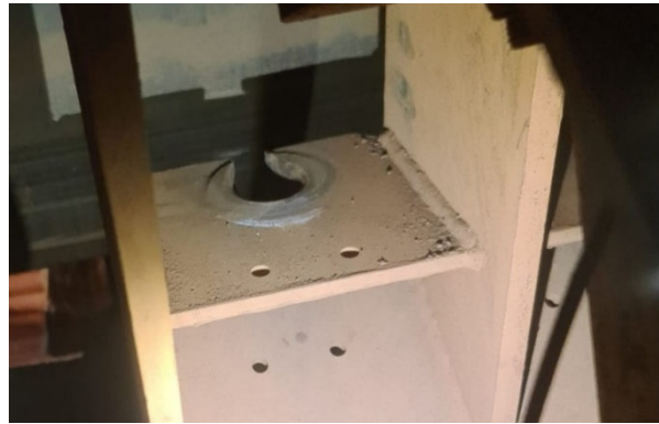
FIG 24 – Roller shaft support plate steel compression.
