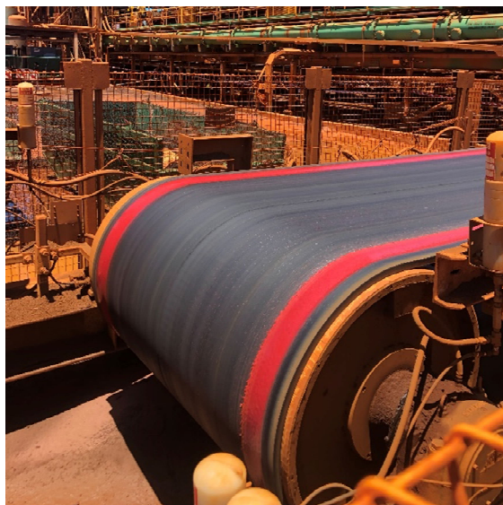
FIG 5 – Belt cover repair system shown here to fill in grooves caused at skirt zones (source: C Uchtman, Wear Systems Solutions).
