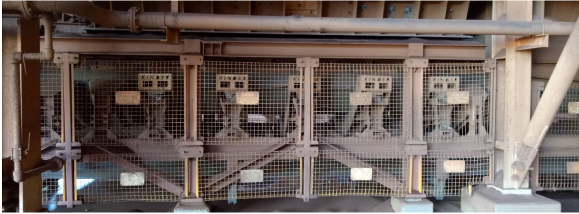
FIG 20 – K-Shield Dynamax® Idlers installed beneath a primary sizer.
