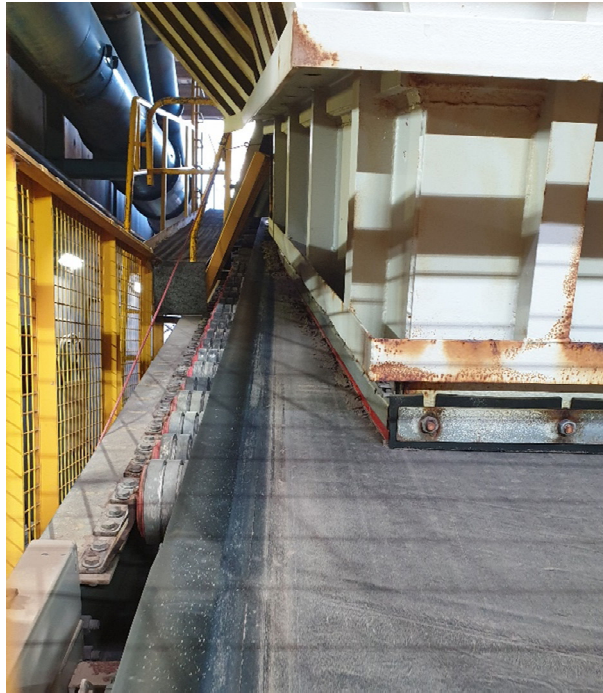
FIG 6 – Tapered chute on a flat belt conveyor system.
