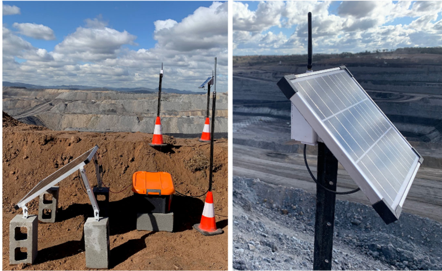
FIG 5 – Gateway and LCS units installed in the active area of a surface mine.
