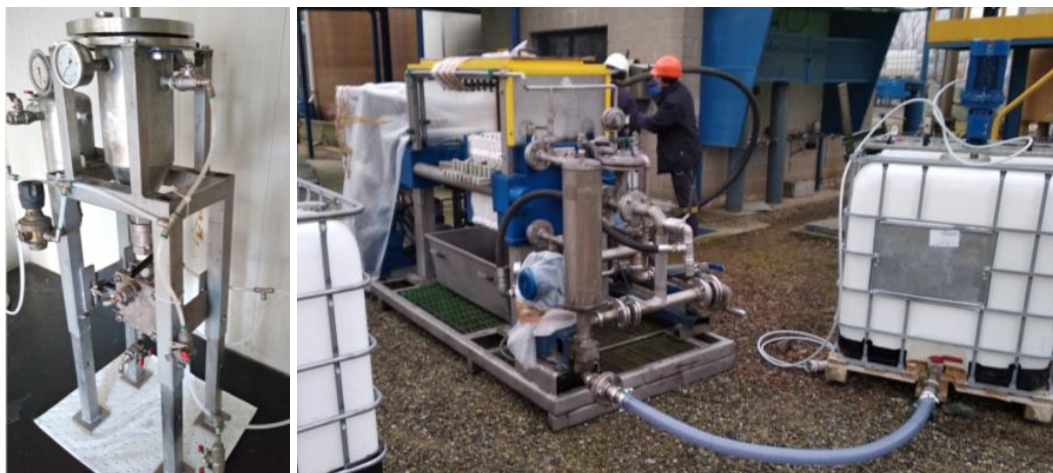
FIG 5 – Laboratory skid and pilot skid.
