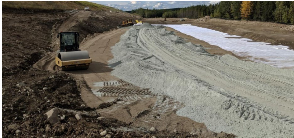
FIG 10 – Drainage at the base of the dam during its downstream expansion using a MLDG.
