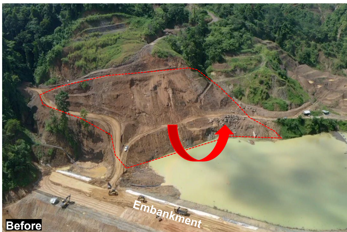
FIG 2 – Upstream batter noted to be potentially unstable.
