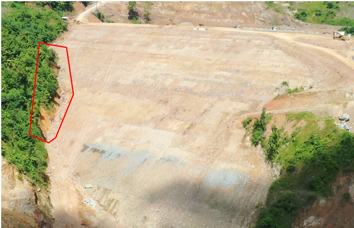
FIG 7 – Significant erosion on right abutment.
