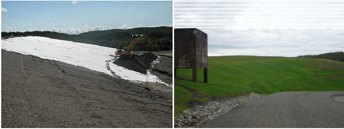
FIG 5 – Mine Waste disposal site during and after construction of its final cover.
