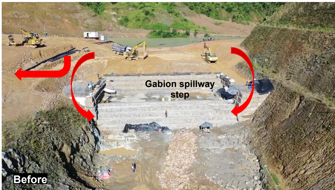
FIG 4 – Gabion spillway walls lower than crest.
