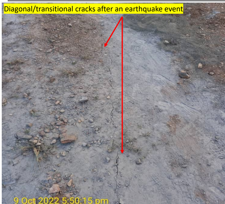
FIG 7 – Pore pressure sudden increase in the earthquake event (top) and irregular scatter and transitional cracks along the dam crest (bottom).
