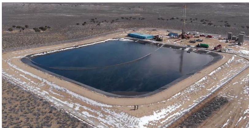
FIG 3 – Double lined produced water pond drained with a MLDG below the secondary liner (groundwater) and the primary liner (leak detection layer).
