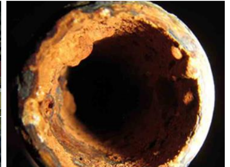
Corrosion inside a pressurized carbon steel air pipe due to wet air
