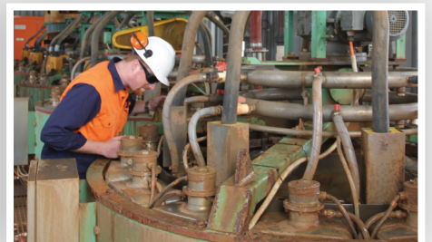
Process Optimisation & Servicing
