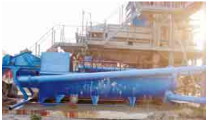
Sand trap in operation
