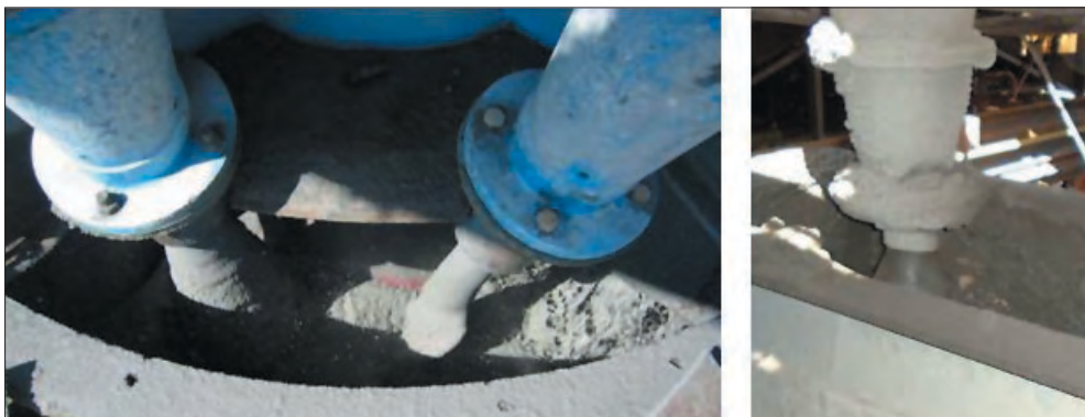
(a) Cover plate removed, revealing a roping cyclone
